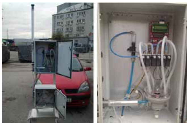
Figure 2 Air sampler for PM_{2.5} fraction positioned at Port of Rijeka
