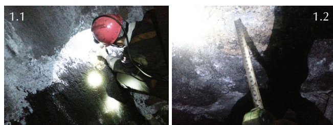
Fig. 1 – Corroded concrete at -355.5 m Slika 1 – Korodirani beton na -355,5 m
