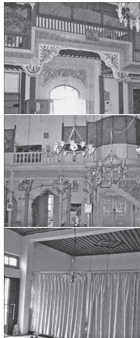
FIG. 1. KOSOVO, PRISTINA, SULTAN MEHMED II MOSQUE, WOODEN LATTICES AND CURTAINS AT WOMEN'S PRAYER SPACE; MACEDONIA, BITOLA, İŞAK ÇELEBI MOSQUE, WOODEN SEPARATORS AT WOMEN'S SPACE, AND CURTAINS FOR WOMEN'S SEPARATION IN BITOLA, HAMZA BEG MOSQUE (FROM TOP TO BOTTOM)
