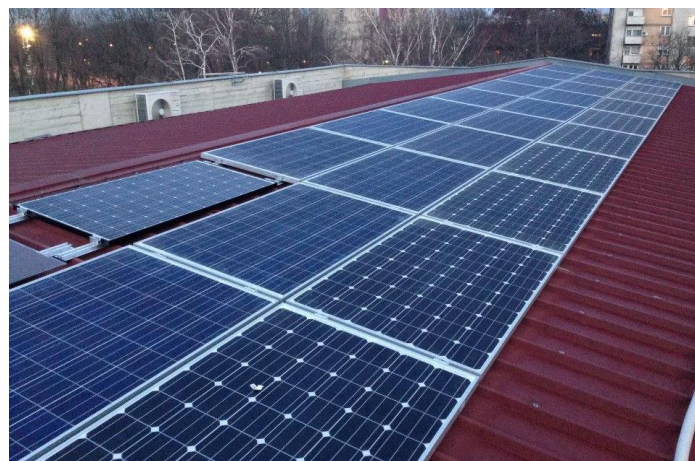
Figure 6 ETFOS 1 PV power plants
