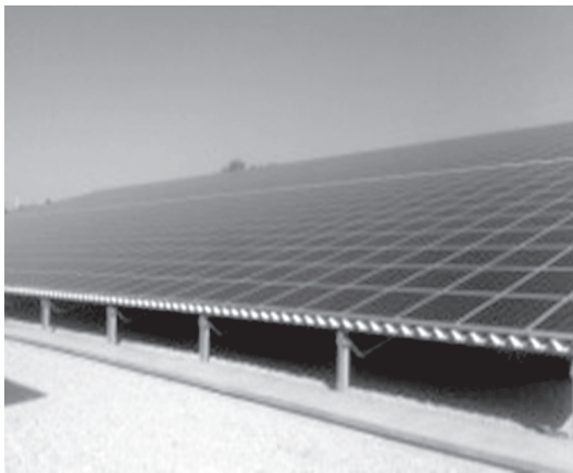
Fig. 1. Solar power plant Domi
