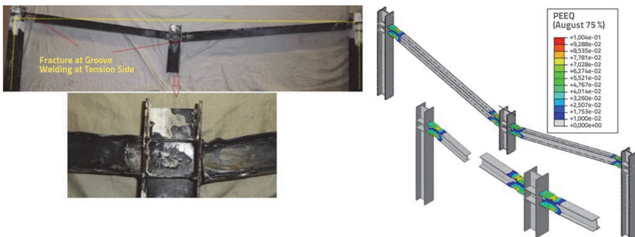
Figure 10. Specimen damage at the end of progressive collapse test and plastic equivalent strain distribution
