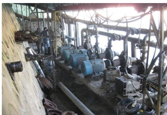
Figure 1. Single-stage raw water pumps installed on an open platform in Srinagar
