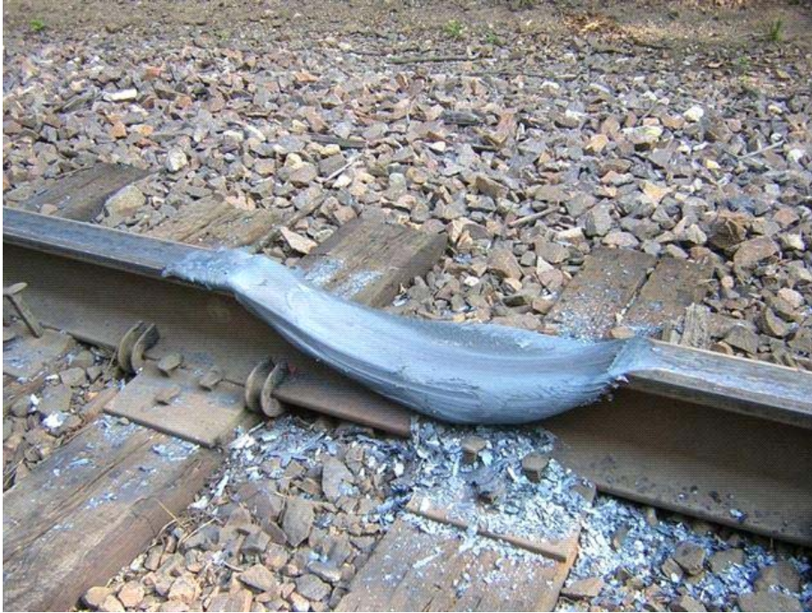
Figure 7: Image showing damage to a rail from adhesive wear action of a spinning rail wheel (photo courtesy Ontario MNR)
