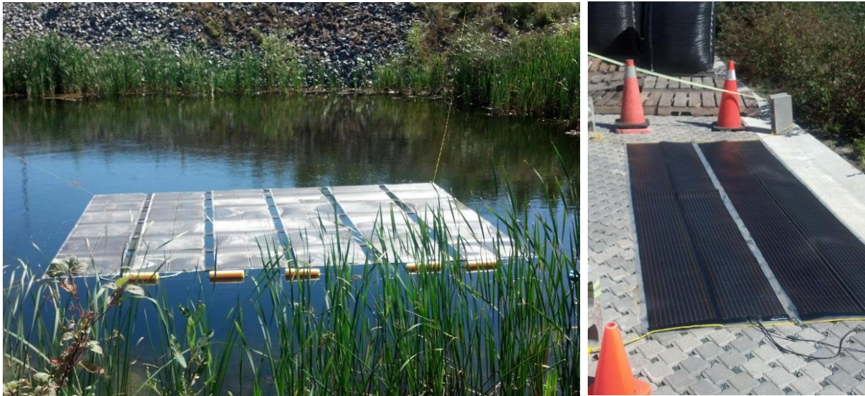
Figure 6-4: 570W_p floating PV array (left) 3 and 190W control array (right)
