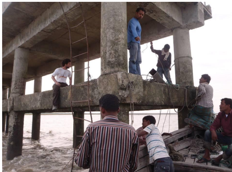
Figure 3. 1: Photo of 1st attempt to install the tide gauge on the eastern coast jetty
