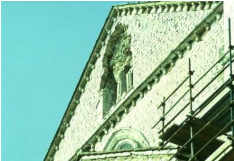
Figure 36 St. Francis Basilica in Assisi: earthquake damage in the transept tympana.
