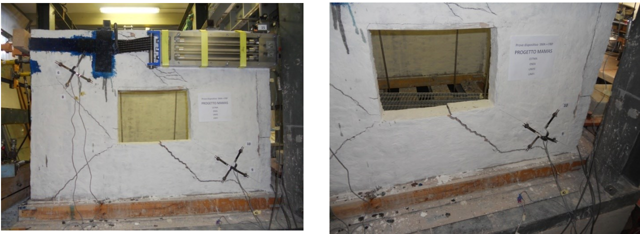
Figure 93 Crack pattern after the execution of the test n. 2 in the hollow wall.
