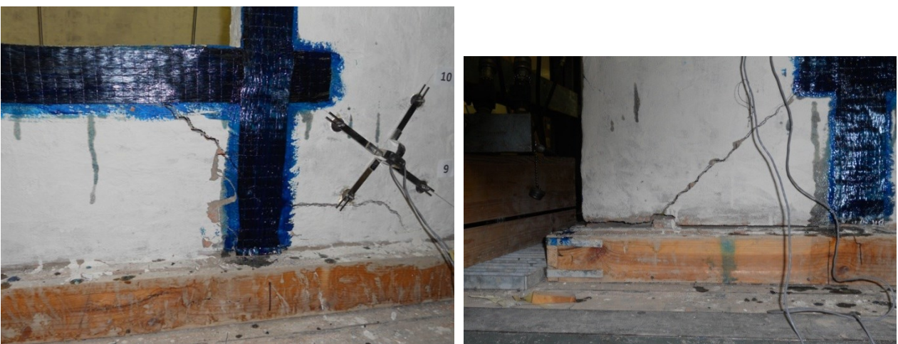
Figure 96 Details of FRP delamination around the hole and detachment of the wall directly loaded by hydraulic rams
