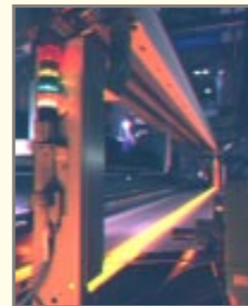
Honeywell-Measurex provides Web inspection systems for Roibox in Aylesford, England.
