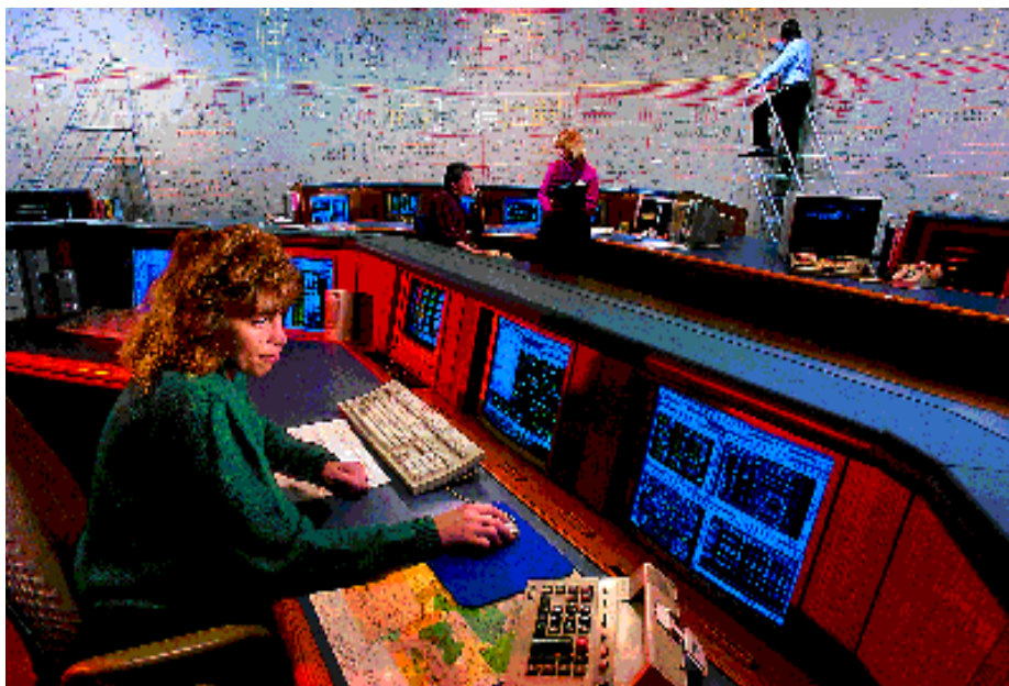
Christine Laskowski of Minnesota Power uses the XA/21™ control system from GE Harris to automatically monitor and control the electric power grid across the northern tier of Minnesota.
