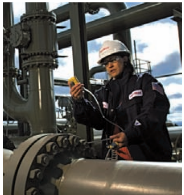
A Piceance plant supervisor conducts routine maintenance activities at the Central Treating Facility, where Piceance Basin gas production is processed for sales.
