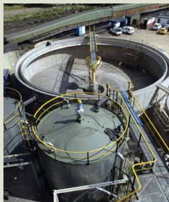
The sulphate reduction demonstration plant at Landau colliery
