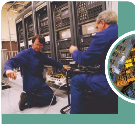
Gateway cabling at the Lille exchange (Northeastern France).
