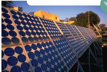
A photovoltaic generator
