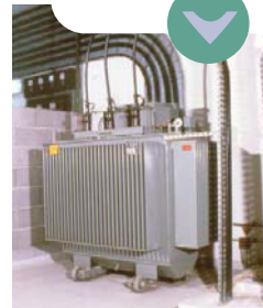
A power transformer incorporating PCB/PCTs
