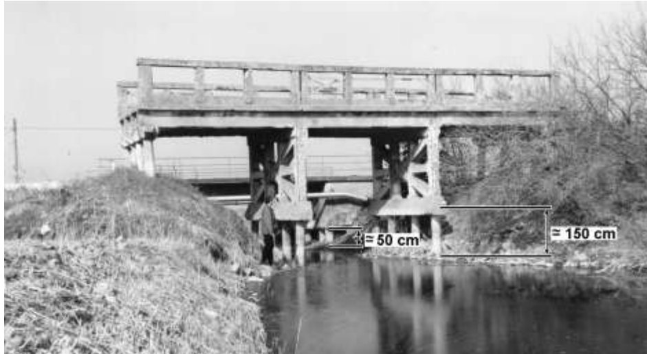
Figure 4. An old bridge constructed in the Twenties whose foundation protrudes about 150 cm owing to land subsidence caused by peat oxidation and groundwater exploitation. In the background, the newer bridge today in use reveals a subsidence of about 50 cm during the last 30 years. The location of the photo is given in Figure 2.
