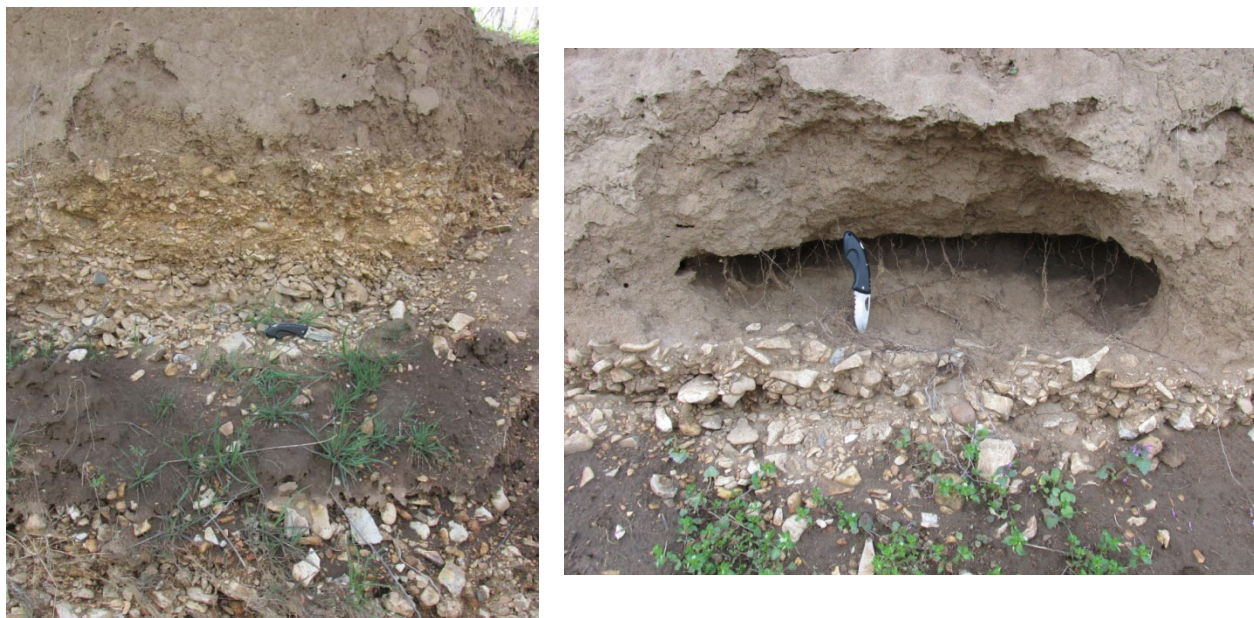
Figure 1. Streambank at the Barren Fork Creek field site including the bank profile (left) and a seepage undercut (right). Note the sloughed material in the bottom of each picture from recent bank failures. These complex alluvial deposits include both clean gravel lenses associated with rapid flow and transport (left) as well as fine gravel lenses that can cause lateral flow and seepage erosion.
