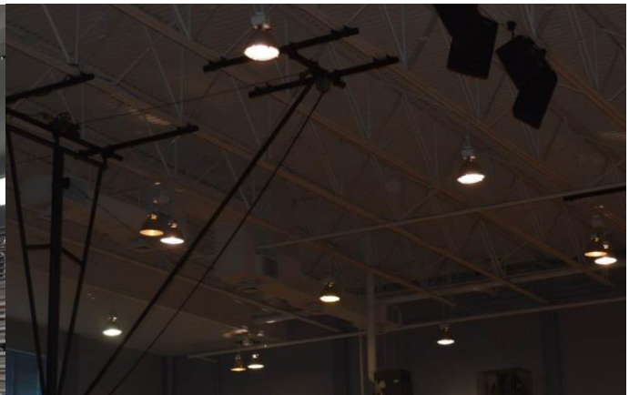
Figure 5.2.1G: Site B – View Gymnasium Lighting
