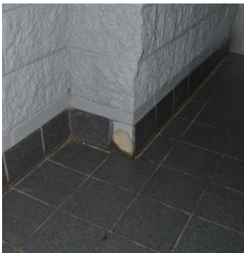
Figure 5.2.1D: Site B – View of Deteriorating Grout and Broken Ceramic Tile Base in Commons Area
