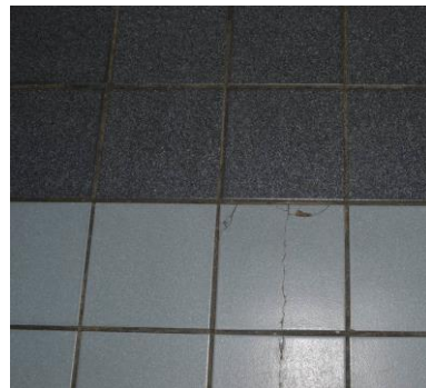
Figure 5.2.1E: Site B – View of Broken Ceramic Tile in Commons Area
