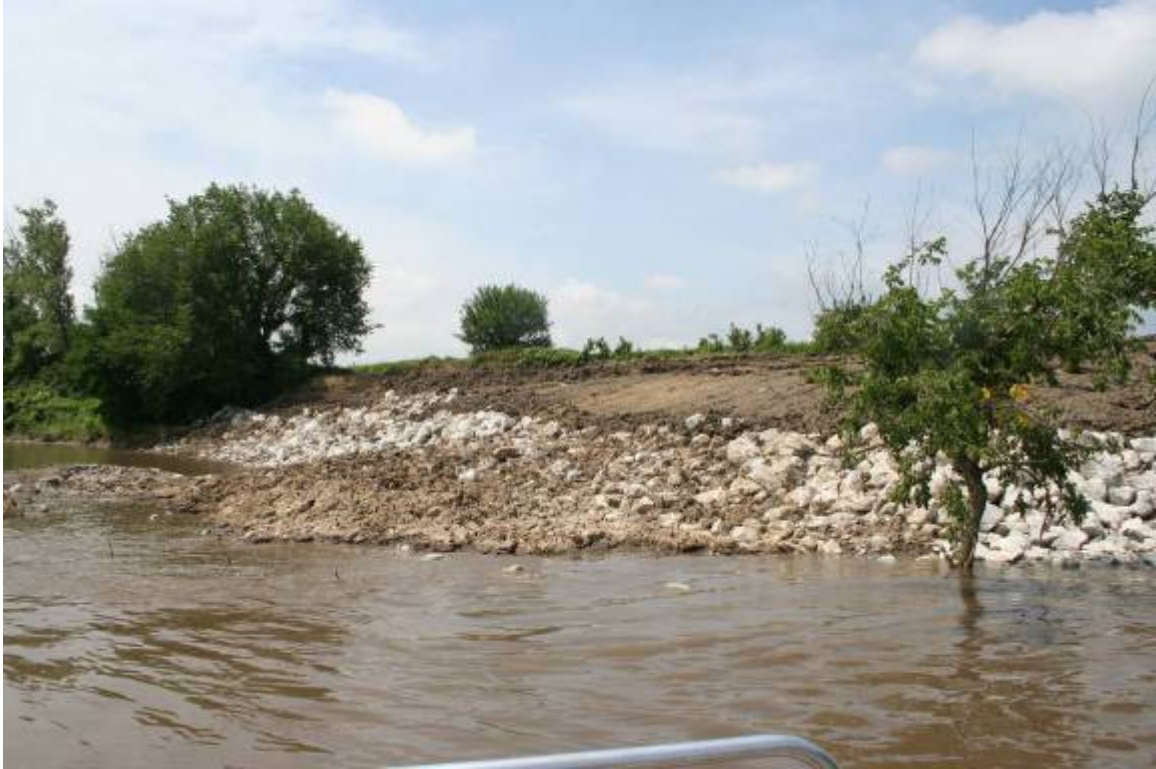
Figure II.3.6. Photograph from July, 2008 of sloughed bank looking downstream.
