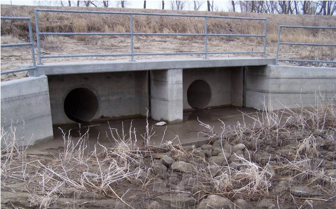
Figure III.1.43. Photo of the Tieville Bend outlet structure without pump operation to facilitate fish movement.
