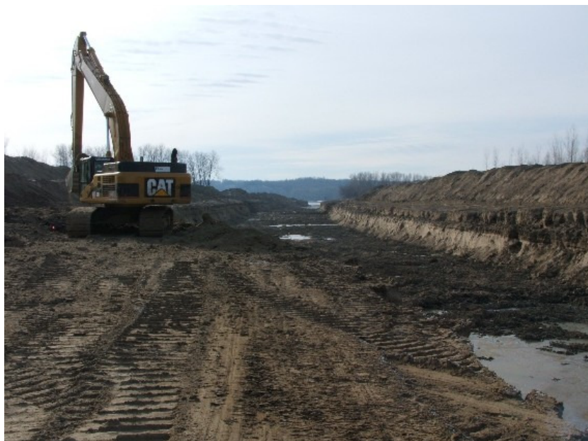
Figure II.12.2. Photo looking upstream from the middle of Tadpole Island Chute while under construction. Photo taken on 12 February 2006 by USFWS, Columbia NFWCO staff.
