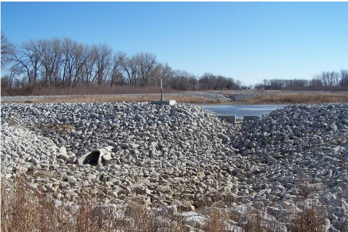
Figure III.1.10. Photo of a weir and culvert below the outlet of the Tieville Bend.
