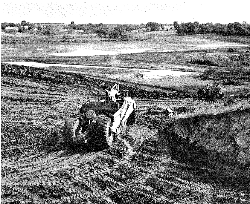
The plans for this reservoir under construction include recreation facilities. Many existing impoundments, like those on the opposite page, were not preplanned for recreation and are either too small or lack access roads, docks, picnic areas and safety features.
