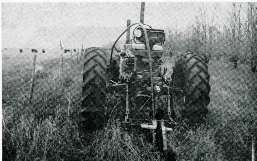
Plastic pipe for carrying stockwater being laid in trench 18 to 24 inches deep and dug by a tractor-mounted subsoiler.
