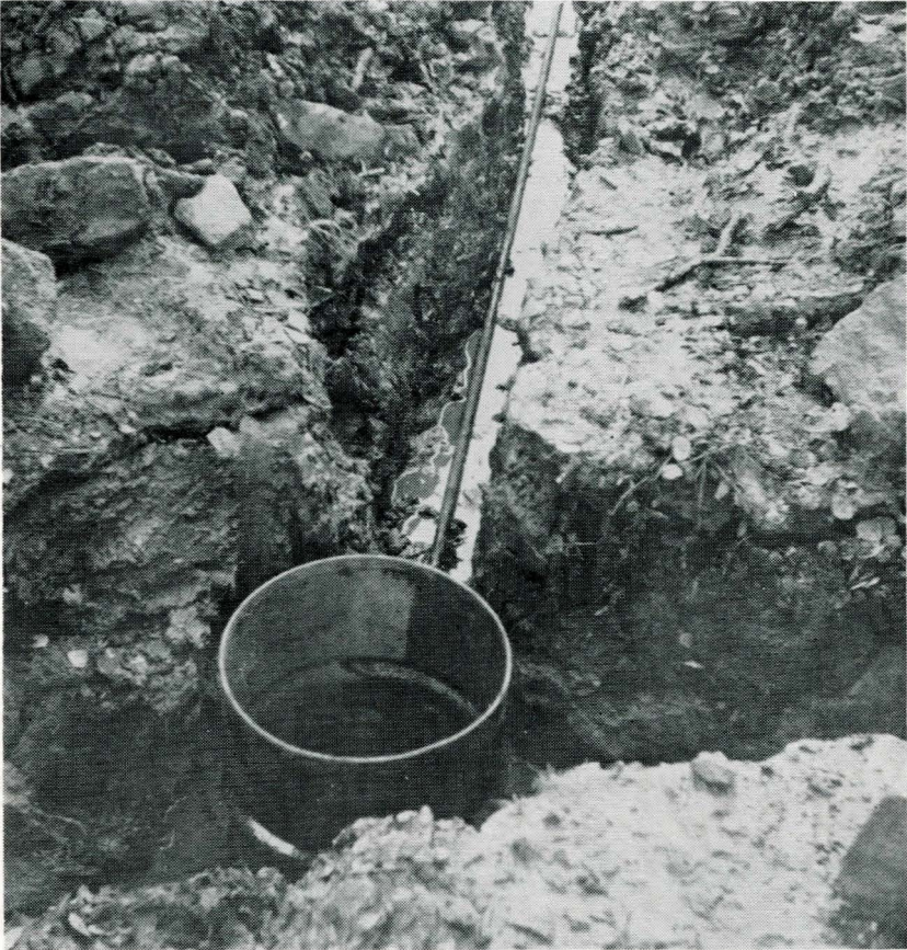
This picture shows installation of collection box and lead-out pipe at a spring site. The box is a 30-gallon barrel perforated around the bottom. The excavation around the box will be back-filled with coarse rock and gravel. (SCS Photo)
