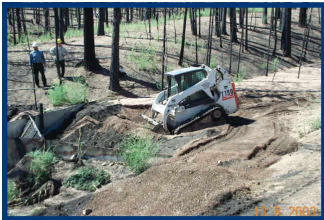
Figure 10.4 —During a short duration high intensity rain event, this research sediment trap was filled. Using pre- and postsurveys, Hydrologist Bob Brown and Engineer Joe Wagenbrenner measure the sediment collected with the help of a skid-steer loader. Research plots are in high severity burned areas of the 2002 Hayman Fire, Pike-San Isabel National Forest near Deckers, CO. (Photo by J.Yost).
