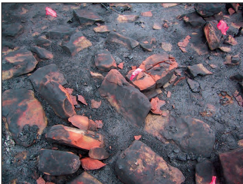
Figure 7-2 —Examples of spalling of sandstone due to heating during the 2002 Long Mesa Fire, Mesa Verde National Park, Colorado: (a) panorama, (b) close up (from Buenger 2003).
