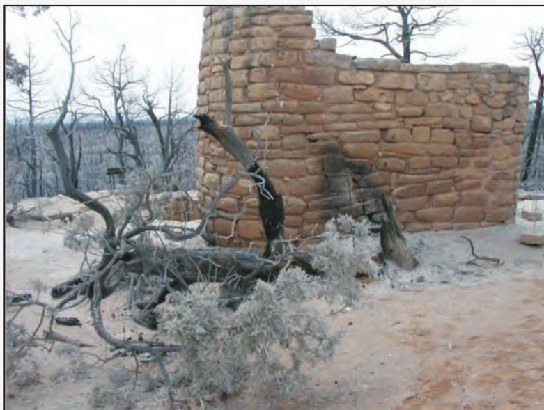
Figure 9S-5c —Damage to a sandstone wall caused by direct flame contact during the 2002 Long Mesa Fire, Mesa Verde National Park, Colorado.
