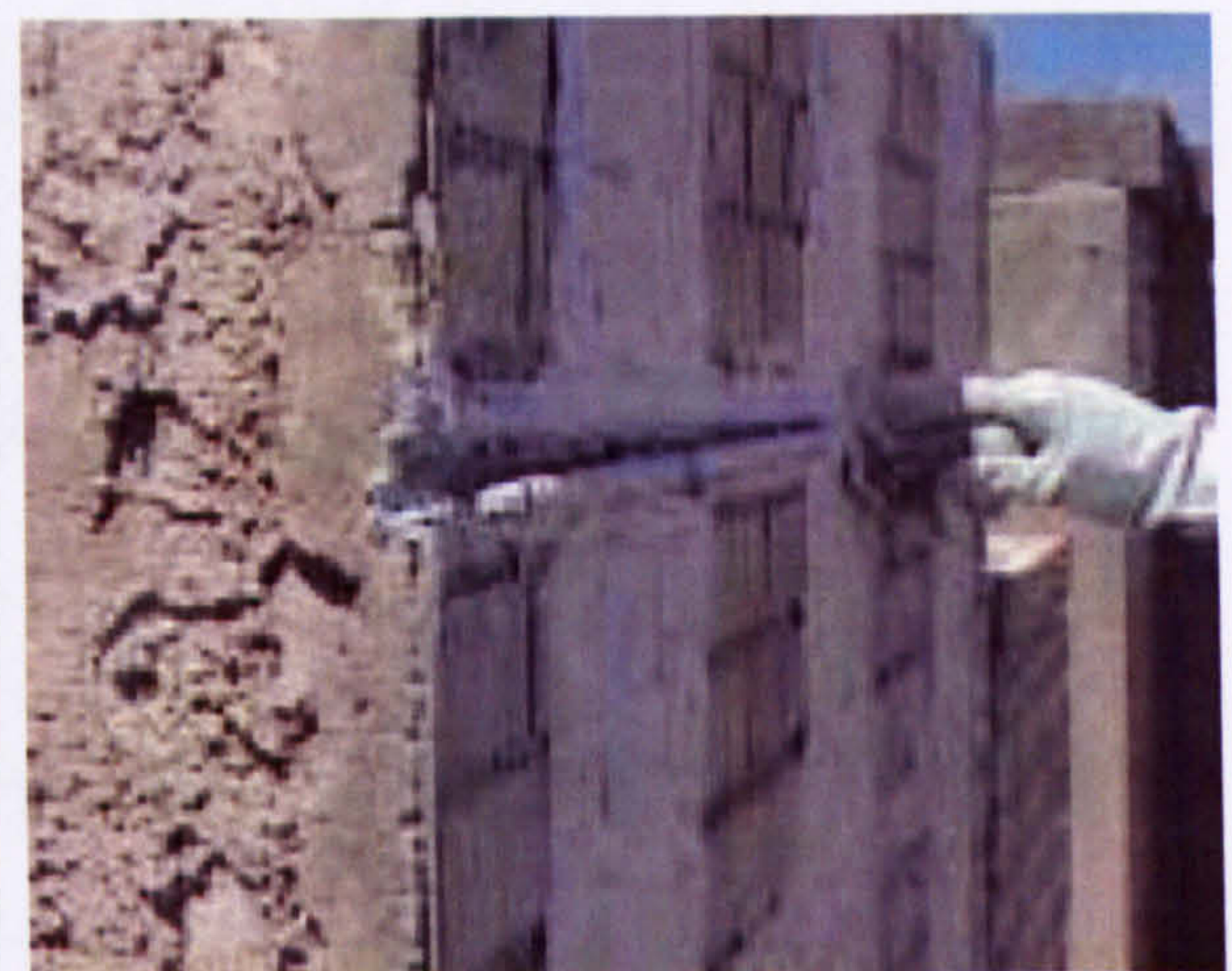
(d) Strengthening and load testing program at Malcolm Bliss Hospital (Tumaialan et al. (1999))
