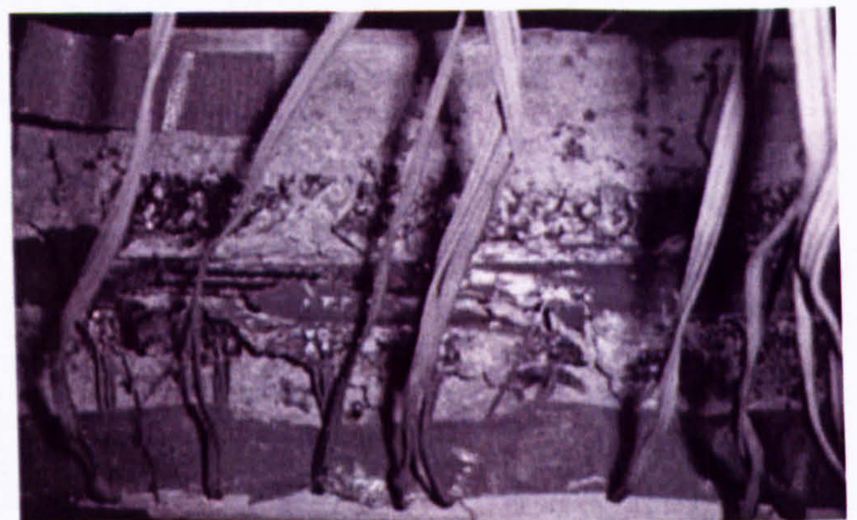
(e) Splitting of the epoxy cover
