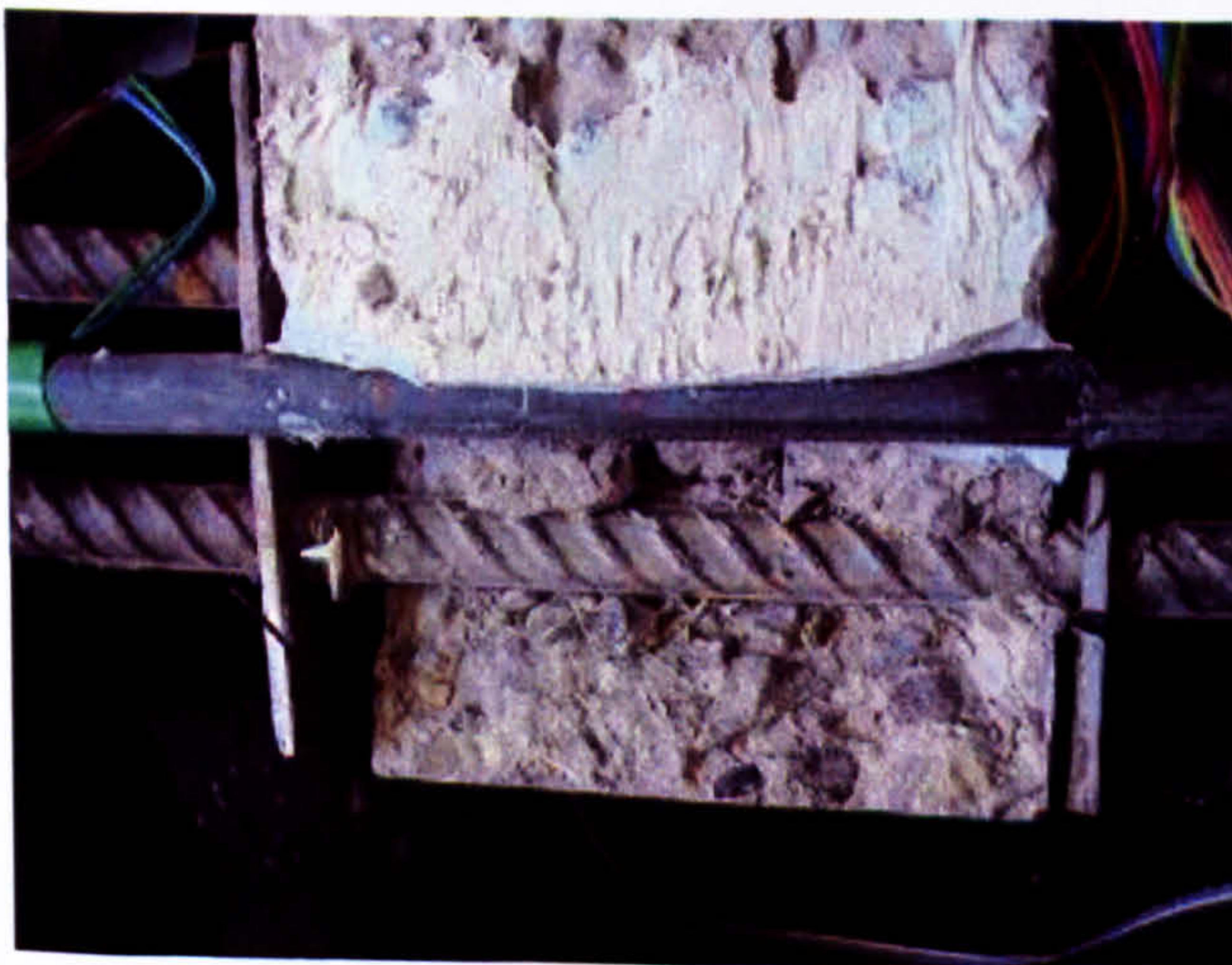
(a) Separation between concrete and adhesive
