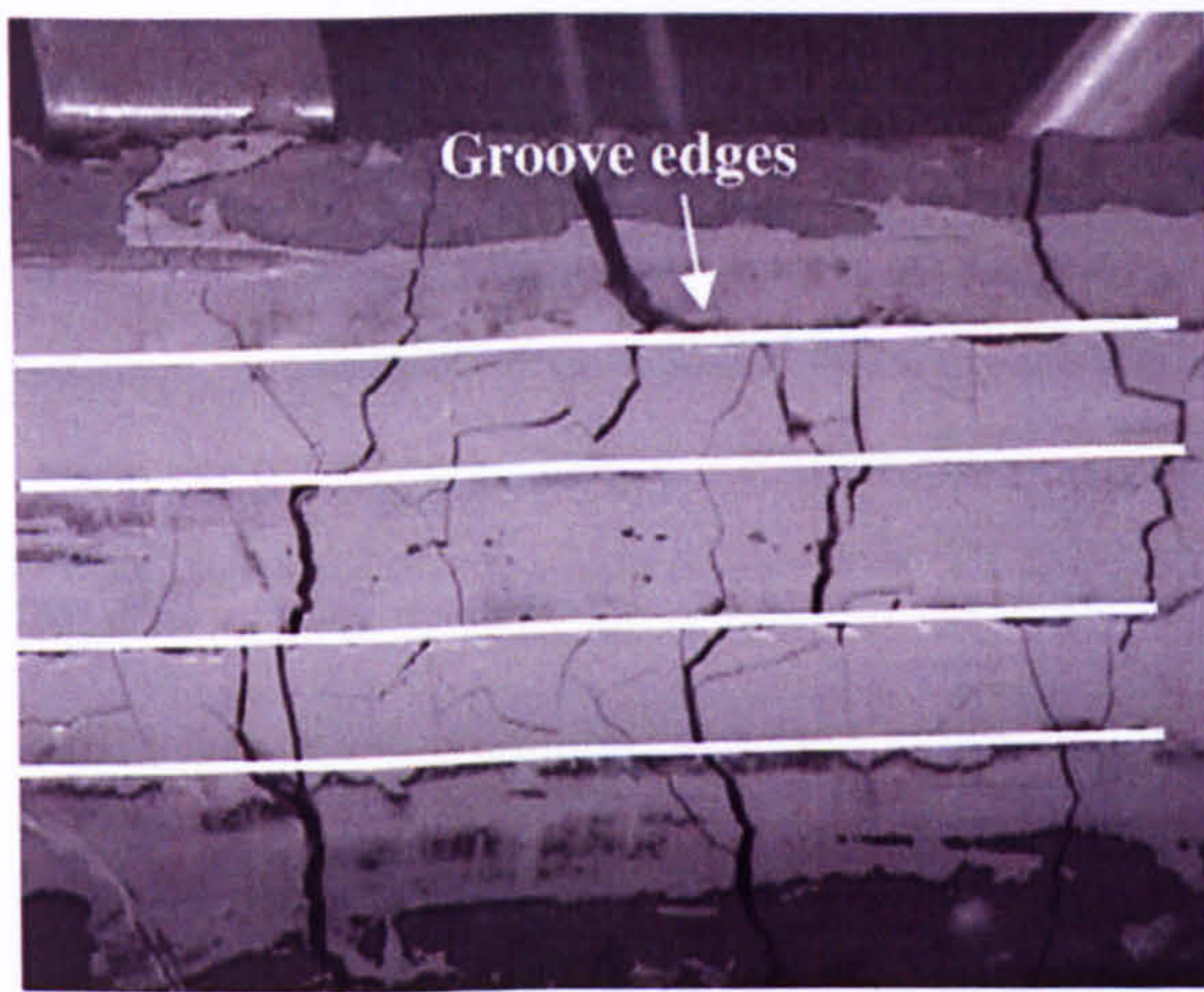
(a) Bar-epoxy interface debonding
