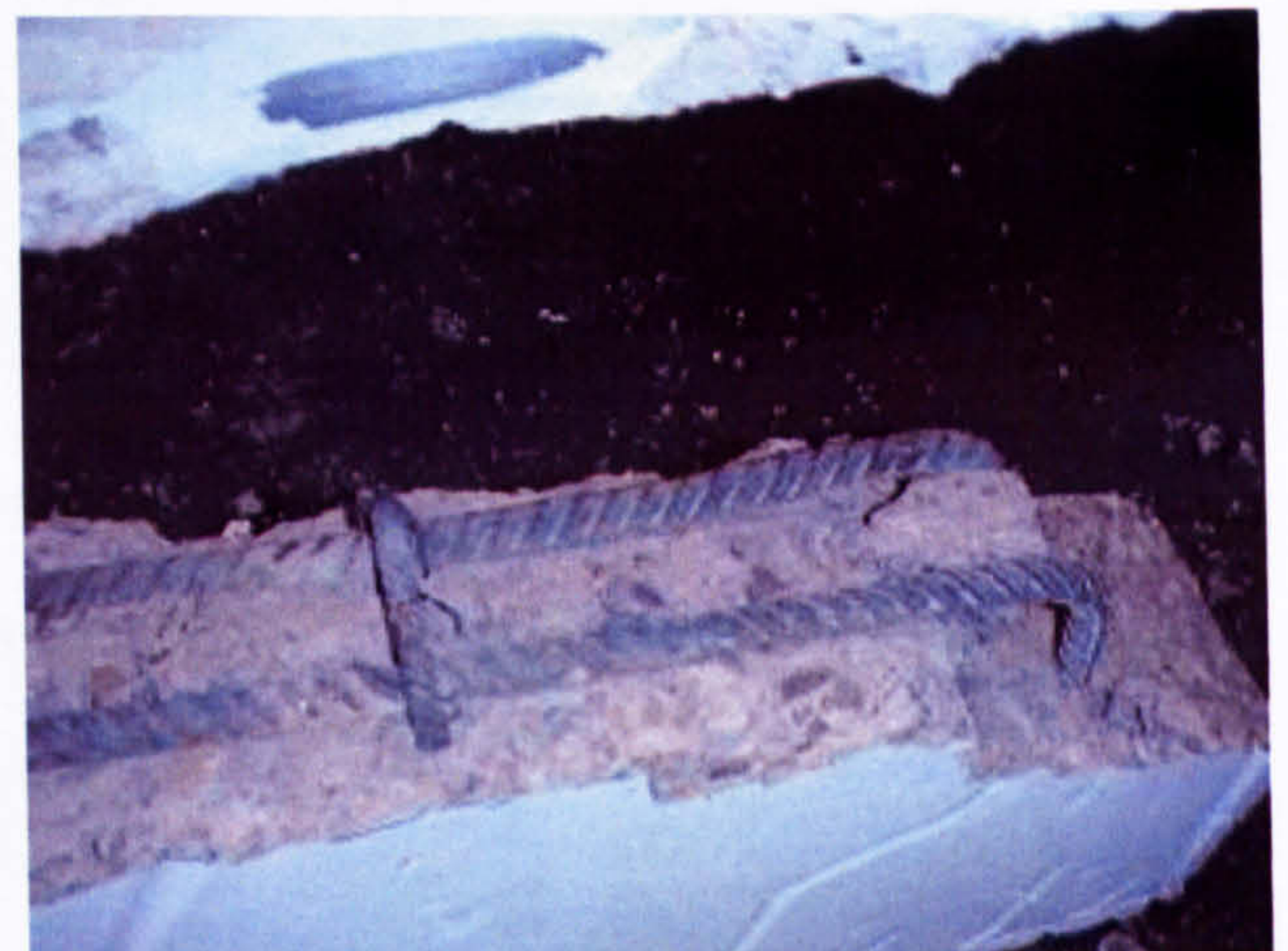
(b) Separation in the cover concrete 2
