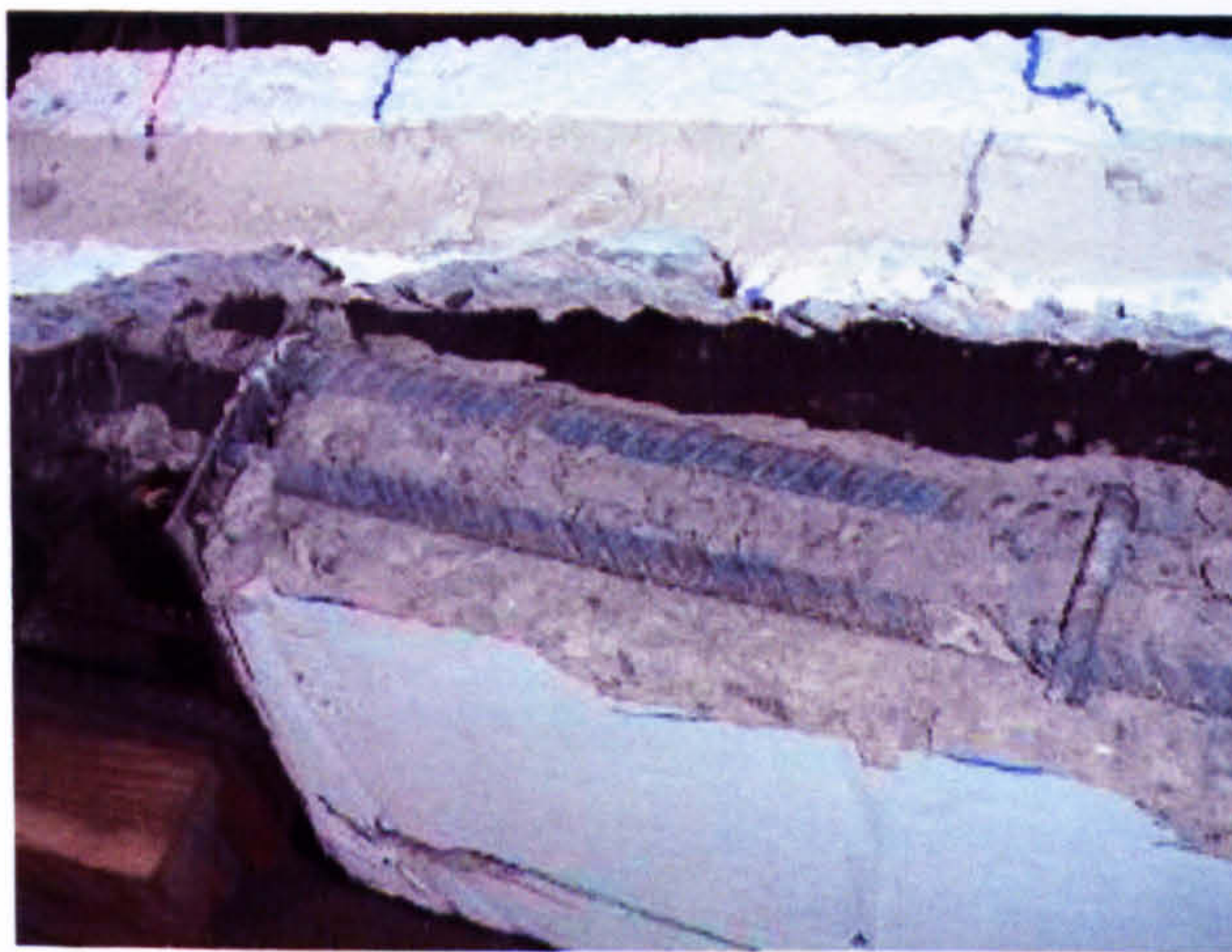
(a) Separation in the cover concrete 1
