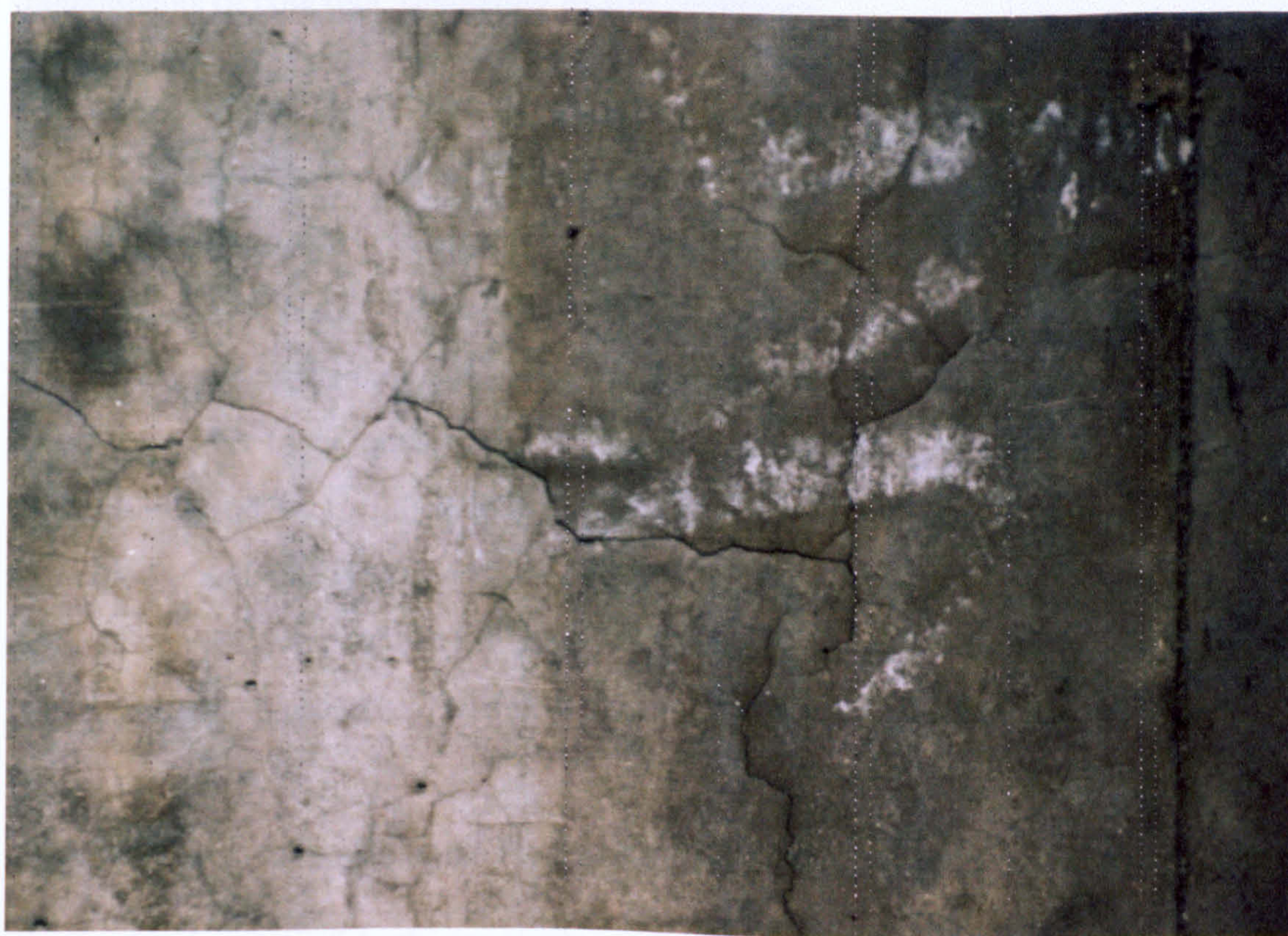
Figure 2.4 Bridge pier in Tianjin, China, affected by both ACR and ASR reactions.
