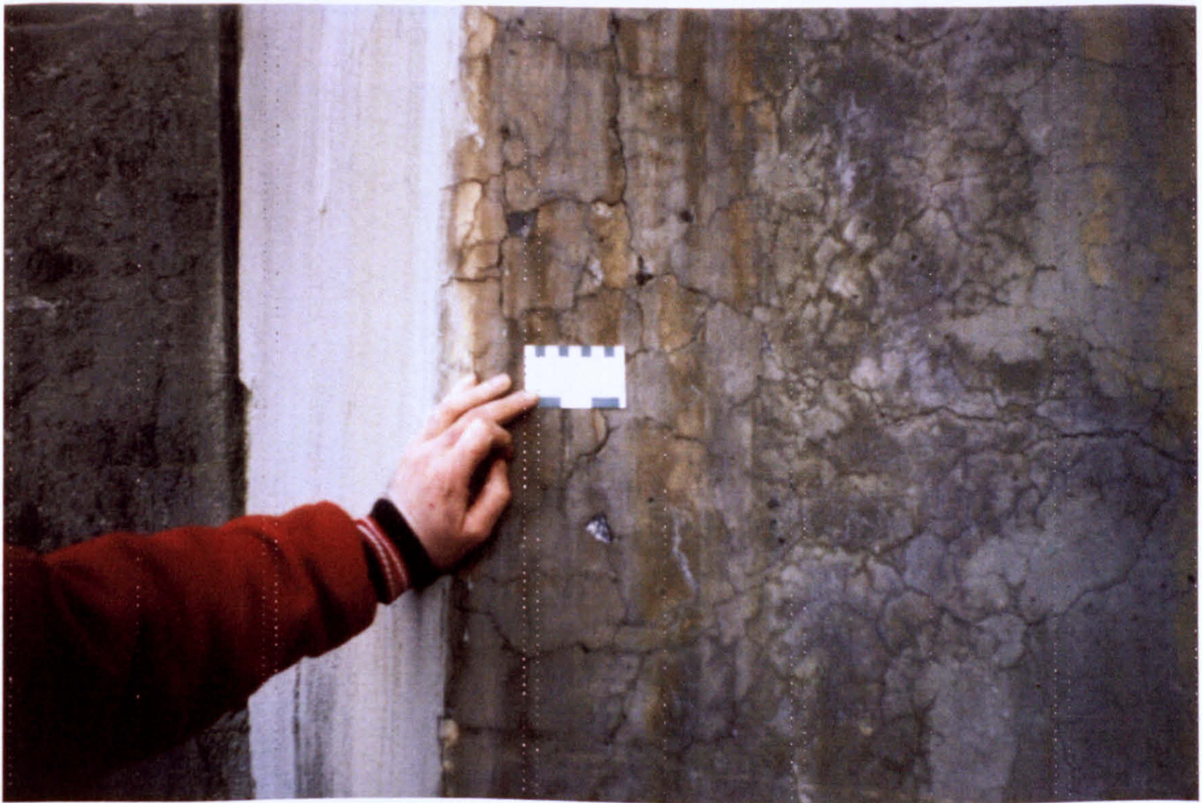
Figure 2.2 An ACR affected concrete bridge showing typical map-cracking. Gananaque, Ontario, Canada, built 1934.
