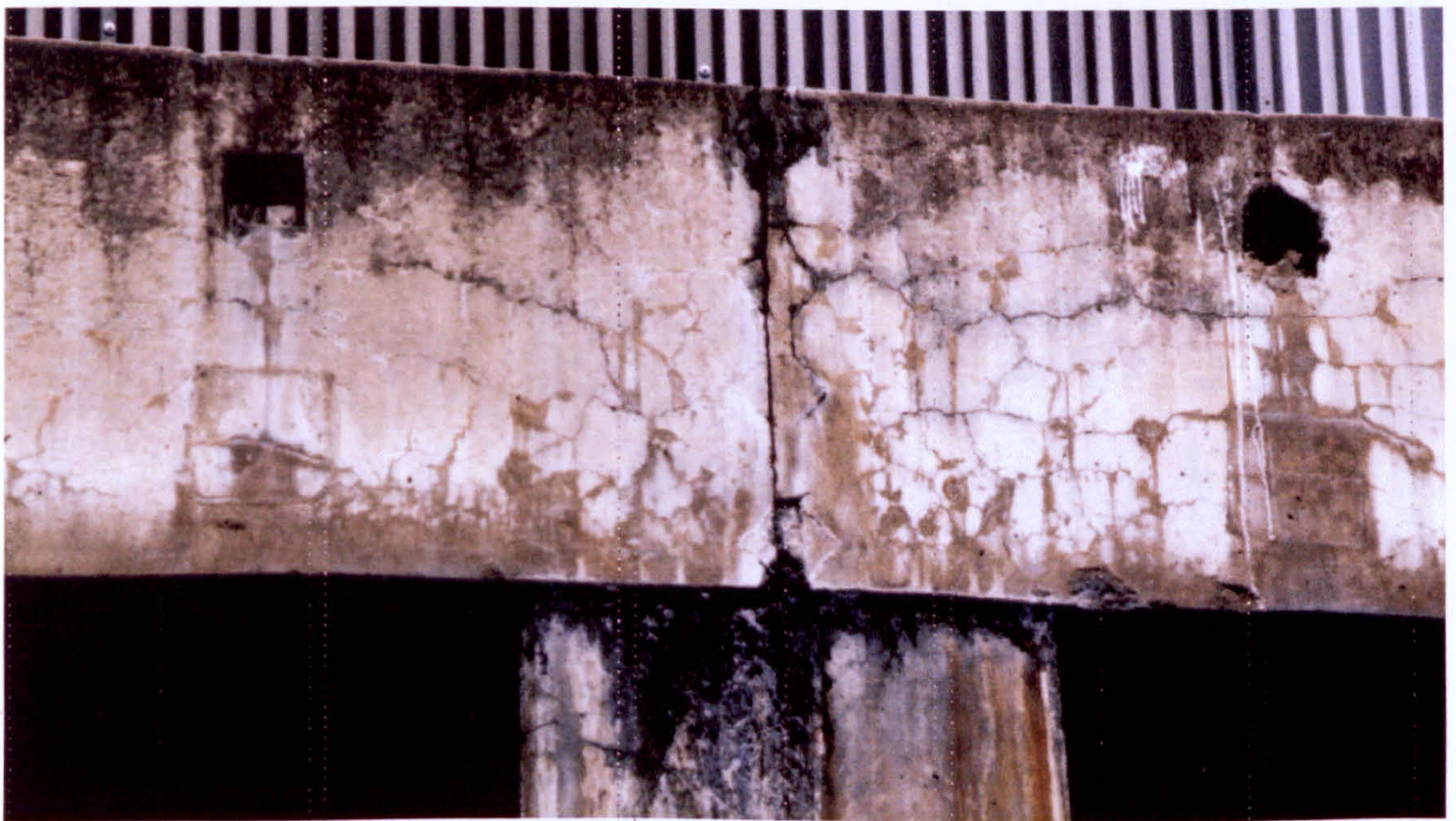
Map-cracking surface of the concrete, close look.
