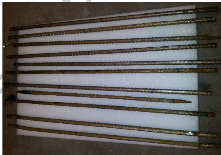
Fig. 3. Corroded reinforcement after cleaning process
