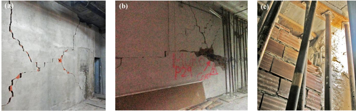
Figure 11. In-plane failures in masonry infill panels: shear diagonal cracking (a), horizontal sliding (b), corner crushing and induced brittle failure of RC column (c) (Calconsa XXI 2011).
