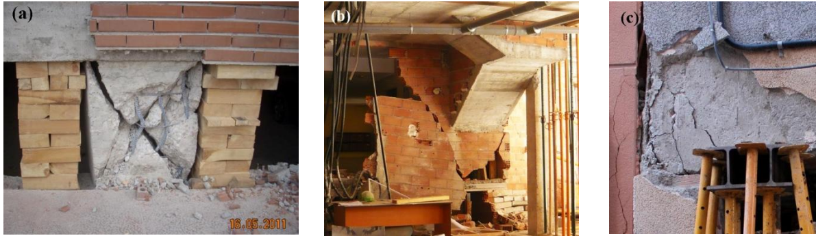
Figure 9. Brittle failure of “squat” column (a) (Vidal et al. 2011), masonry staircase (b), beam-column joint (c).
