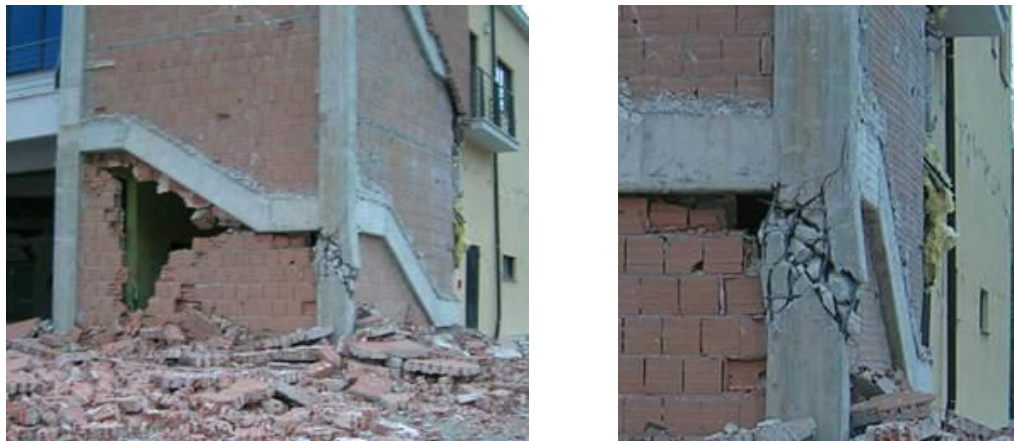
Figure 9. Shear failure in squat columns of the staircase
