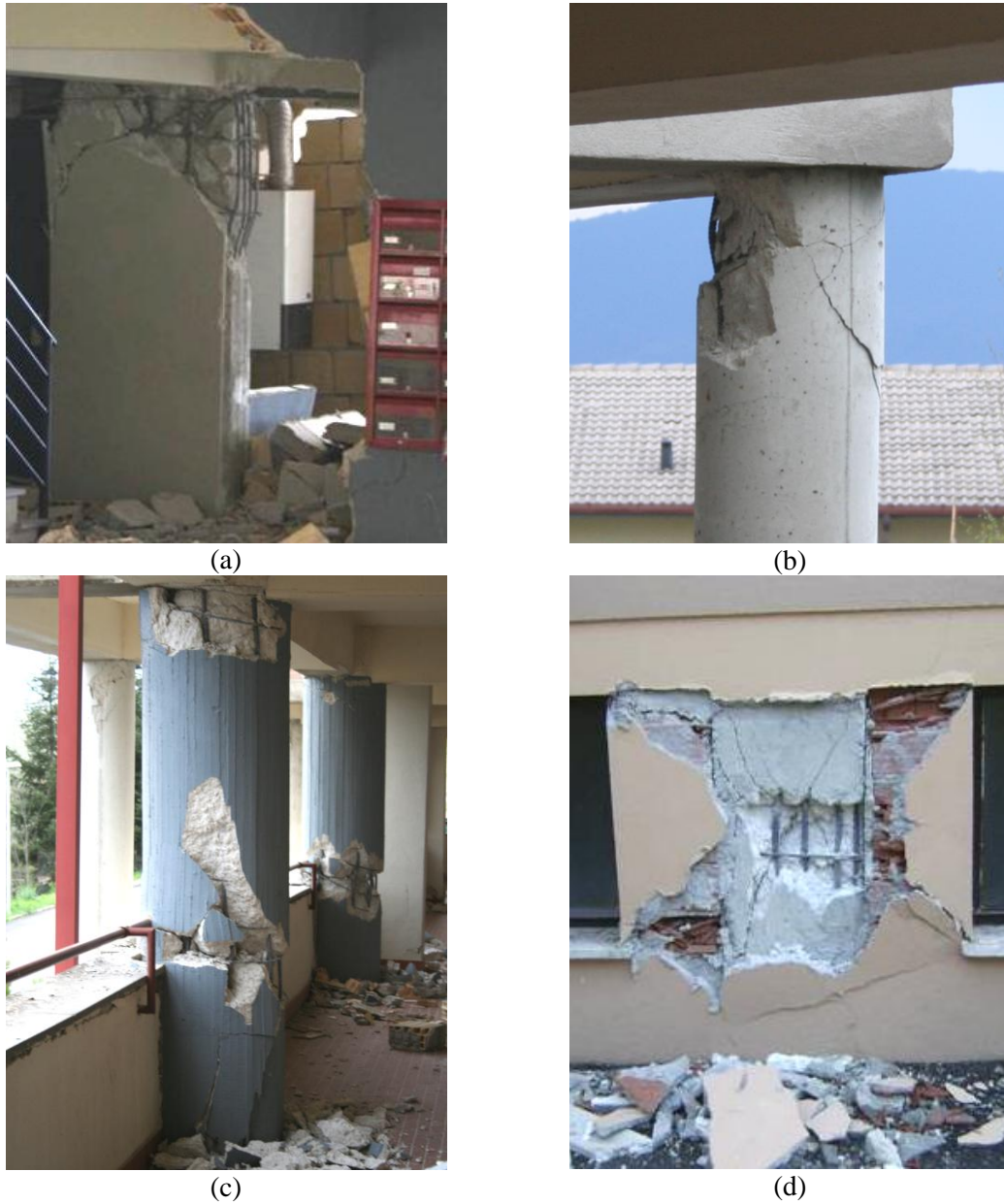
Figure 8. Shear failure of: (a) rectangular and (b) circular (b) columns, (c) column adjacent to partial infilling panels, (d) squat column adjacent to basement level concrete walls
