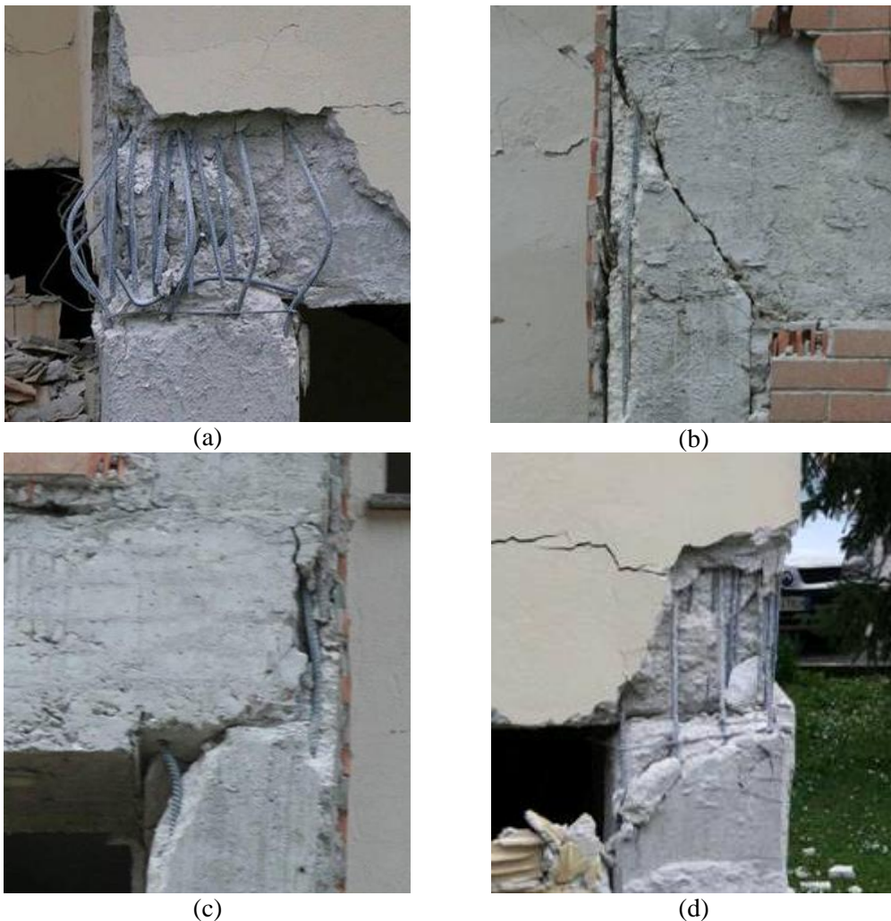
Figure 11. Joint failure with evident (a) longitudinal bar buckling and (b) diagonal cracking failure in concrete joint panel; (c) (d) failure mechanisms at joint – column interface surfaces
