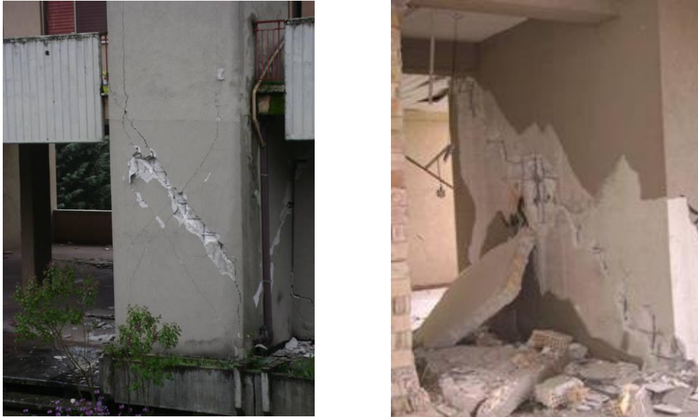
Figure 10. Failure in reinforced concrete walls
