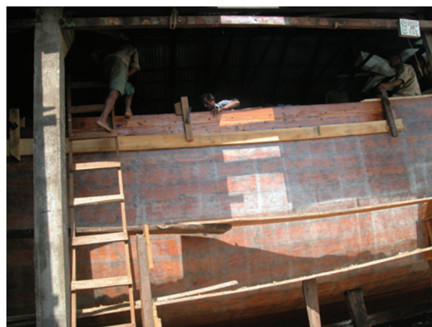
Fig. 2. A multi-day deepsea trawler under construction at the boat building yard, Malpe
