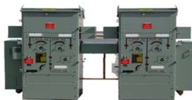
Figure 5. Typical Arrangement of SF6 Ring Main Unit
