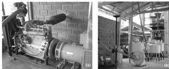
Figure 1. RICE-generator (a) and (b) Gasifier installed in Necoclí (Colombia)
