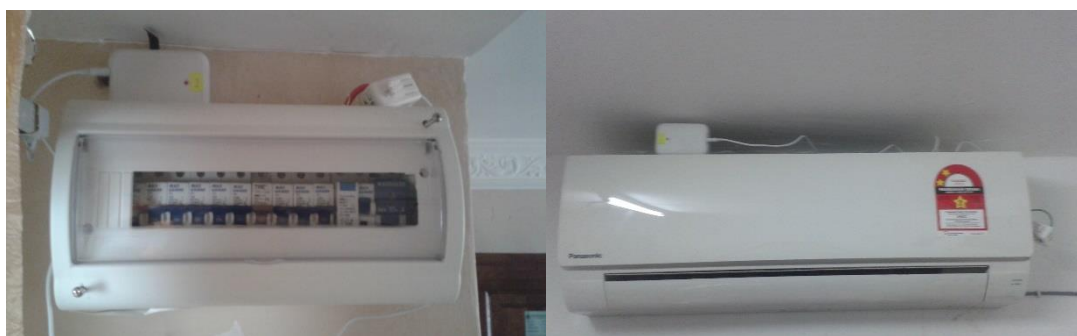
Figure 1. Installation of power monitoring device at a miniature circuit breaker (left) and an air conditioner (right)
