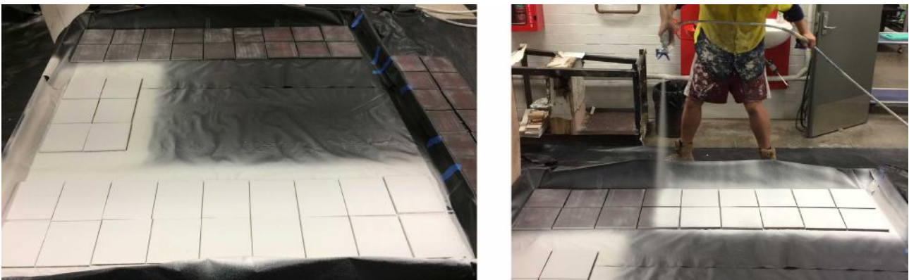
Figure 3.12: Application of the intumescent coating on steel plates using airless spray equipment.
