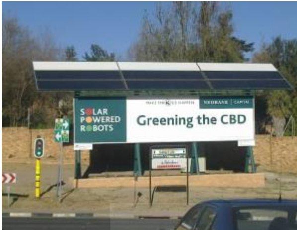
Figure 20: Solar-powered traffic lights
