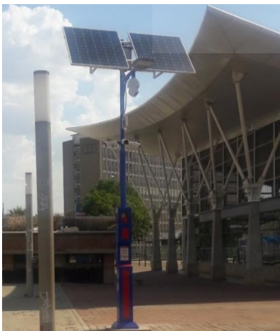
Figure 18: Solar powered CCTV
