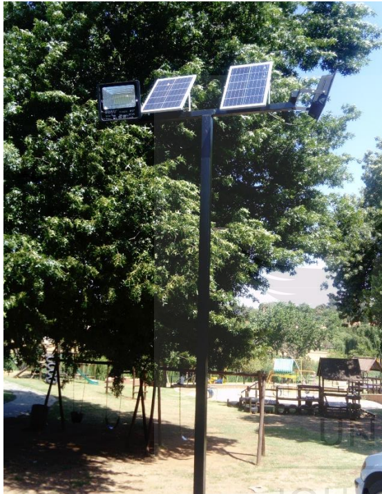
Figure 19: Side-walk solar powered street lamps
