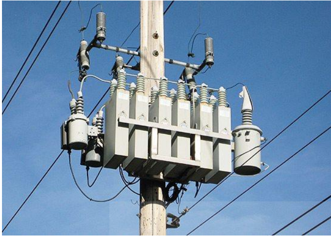
Figure 12: Distribution capacitor bank
