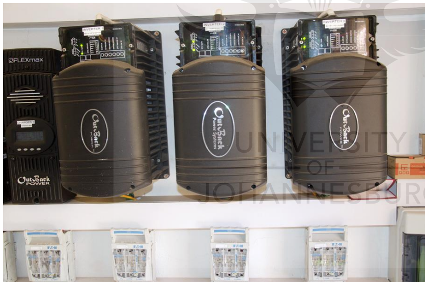
Figure 15: Smart Solar PV system
