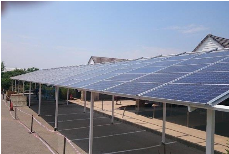
Figure 9: Solar park roofing in GeoSolar premises, Johannesburg
