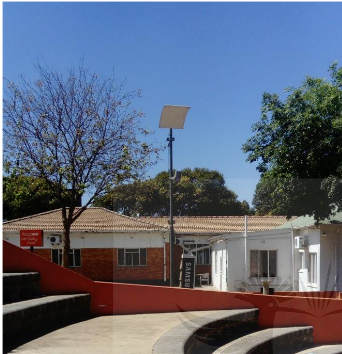
Figure 11: Solar powered lamps in Doornfontein Campus, University of Johannesburg
