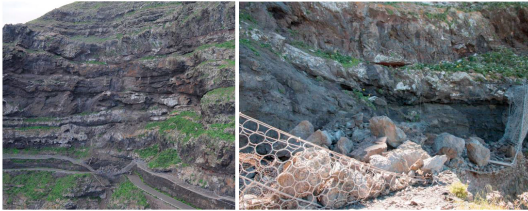
Figure 6. Examples of rockfalls affecting the GC-200 road during the event that occurred on 9th December 2016 (credits R. Sarro and J. Naranjo).
