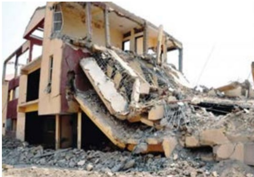
Figure 3: Another view of the building showing the wreckage. Source: [18].
