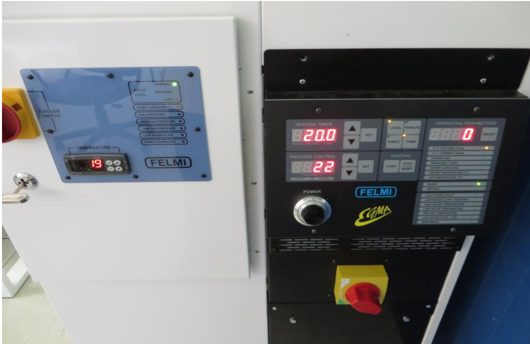
Figure 34: Egma 30R generator panel control
