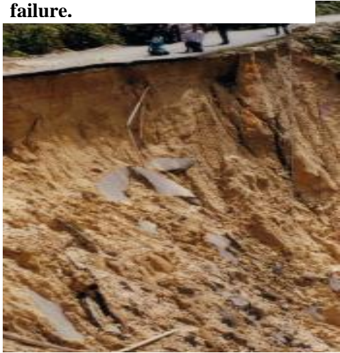
Fig. 5 : Major road embankment failure.
