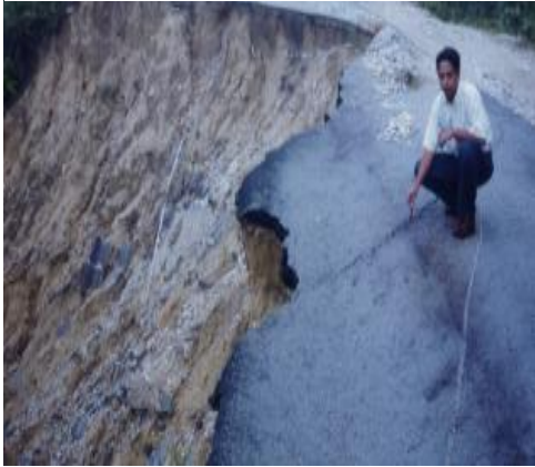
Fig. 6 : Another view of the road embankment failure. The road was totally impassable to vehicles.
