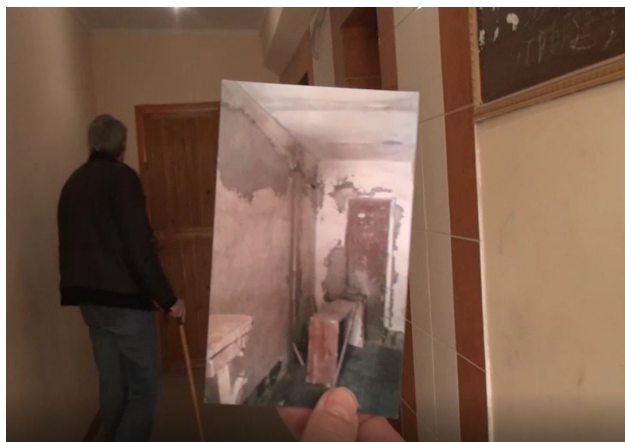
Figure B.7: The Problem of Dilapidated Common Property in Kherson Region
