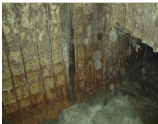
(a) Corrosion prior to repair in 1999
