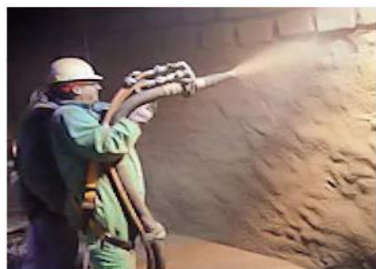
(d) Rehabilitation of pipelines and tunnels in place by shotcrete added with ConShield
