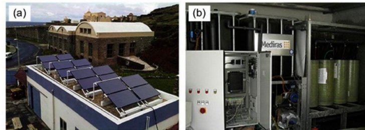
Figure 9. MEDIRAS project MD pilot plant installed in Pantelleria, (a) PV systems; (b) desalination plant pilot obtained from Viola [16], with permission Licensed under CC BY-NC 4.0 from International Journal of Heat and Technology, 2016.
