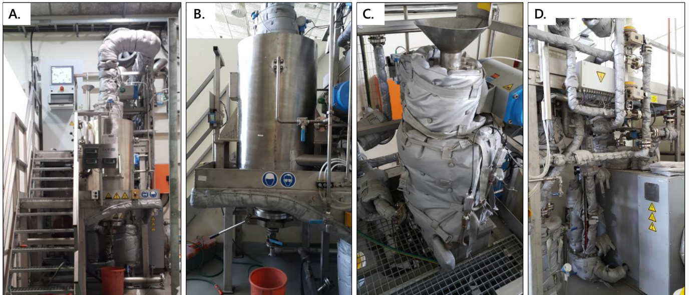
Figure S4.5: Illustration of (A) automated pilot-scale steam explosion unit with 19-L reactor, 100L-discharge tank, and 40 bar steam boiler (B) 100-L discharge tank, (C) 19-L reactor equipped with insulation jacket, steam delivery pipelines and 40-bar steam boiler
