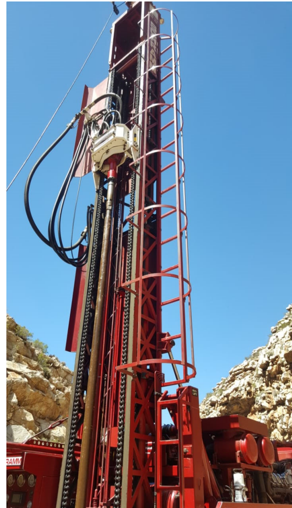
Figure 32: The tower of an air-pressure drill. Source: Private archive of Dirk Steyn of the farm De Oude Muur, Montagu.
