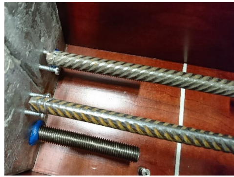
Figure 4. Top view, close-up of the bottom of the formwork, note the white plastic ruler perpendicular to the reinforcement bars to create the notch.
