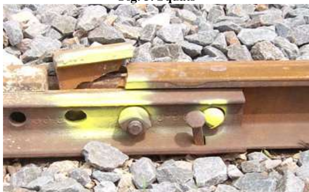
Fig. 4. Broken end rail
