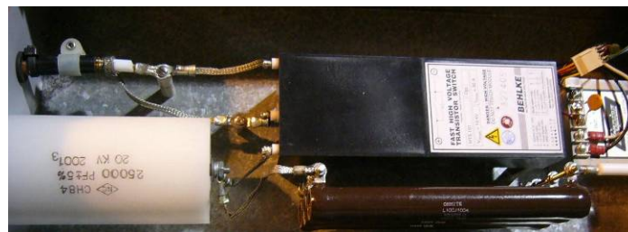
Figure 9. High voltage switch
