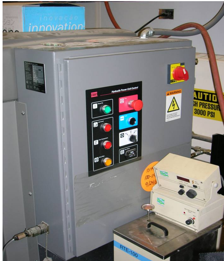
Figure 15. Hydraulic pump and chiller system.
