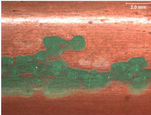
Figure G.72. Digital picture of the interior of copper recirculation pipe.
