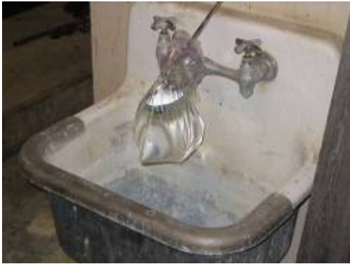
Faucet leaked overnight and filled the bag.
