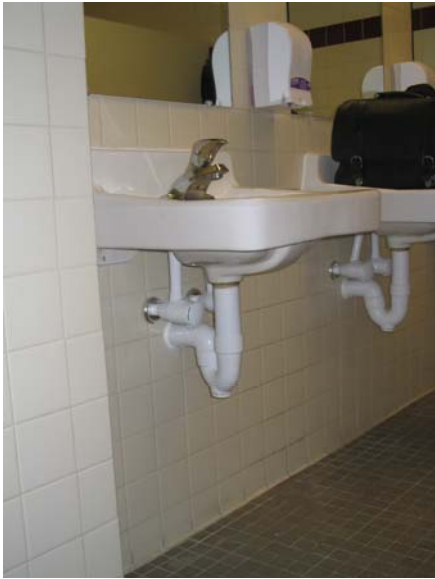
Sink sampled for building 641, and for the sequential sampling.
