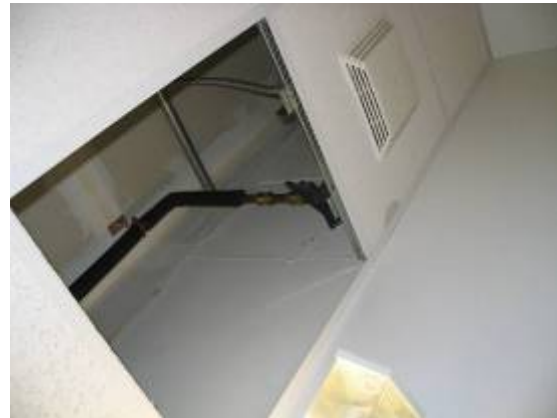
Location of the pipe sampling, above the ceiling over the sink and urinal.
