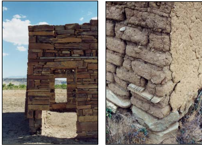
Figure 2.16. Pueblo Construction Materials. Pueblos were constructed of stone or adobe block depending on material availability (Ballweg, 2005).
